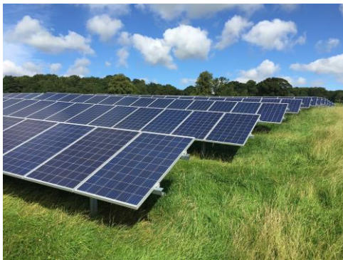
Fig 3 Ground mounted piled single panel table
